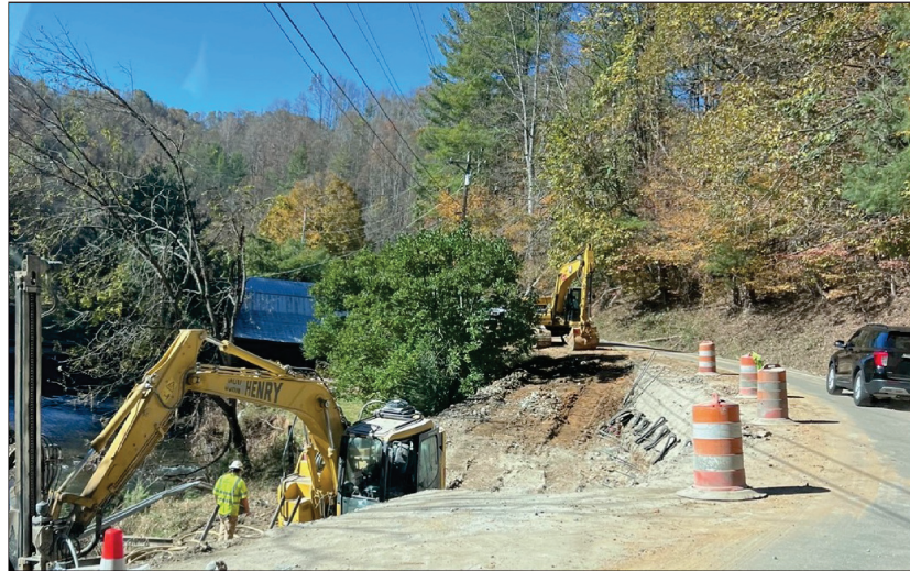
Figure 1: Road Repair Following Hurricane Helene, North Carolina
