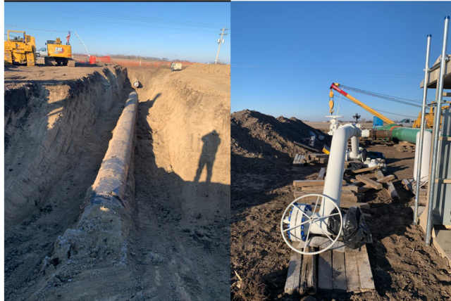
Figure 1: Pipeline and Safety Shut Off Installation on the DGRS farm outside Glenville, Nebraska
