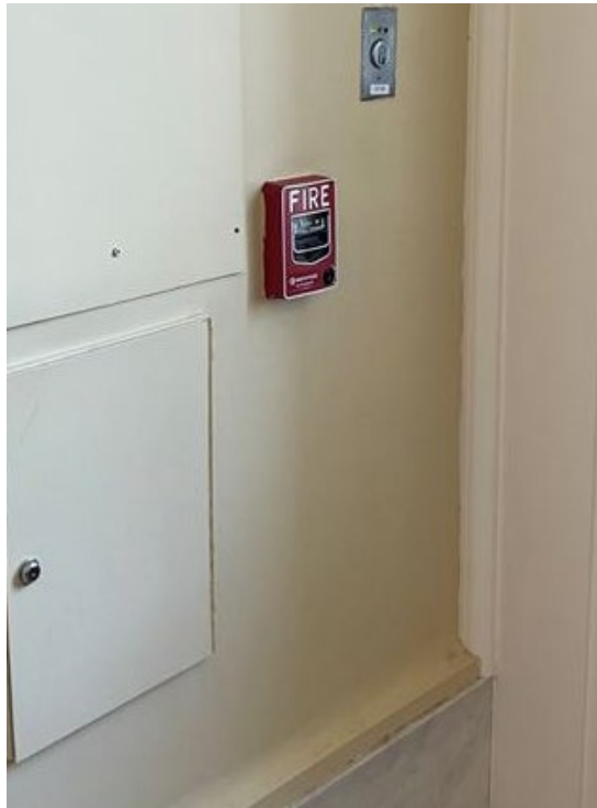
Image of Fire Alarm Station 27
